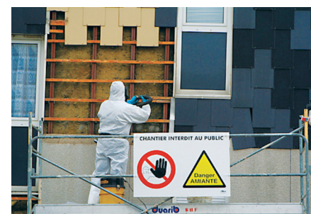
Fig. 2.13.2 Asbestos insulation is common in buildings and presents a hazard when disturbed during demolition. Protective clothing must be worn to avoid contact with asbestos fibres.
